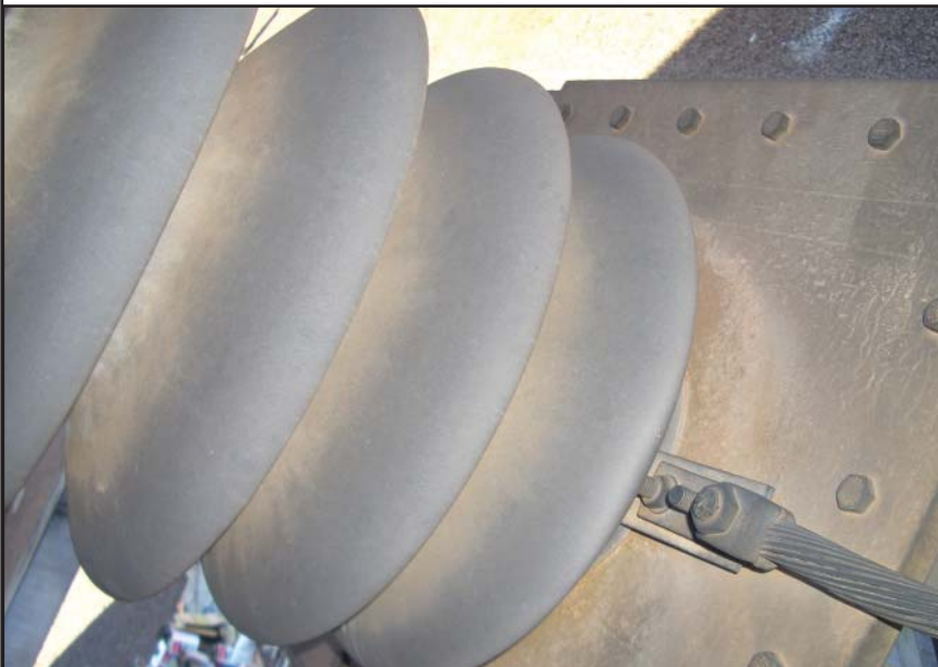
A \pm 600 kV HVDC post insulator at Itaipu, Brazil, heavily contaminated 5 years after Si-COAT application.
